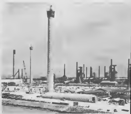
April 1970: Several foundations completed for HDS units, two completed, one small tower installed.
